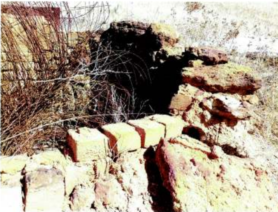
P13670 Lime Kilns, Howatharra Kiln 1: view showing detail of perimeter wall. L Gray 15 April 2010
