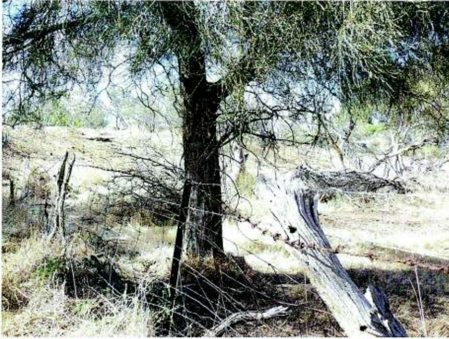
View looking southeast showing the remnants of a culvert in the side of the alignment formation (left) with concrete formed side catchment walls. April 2010.
