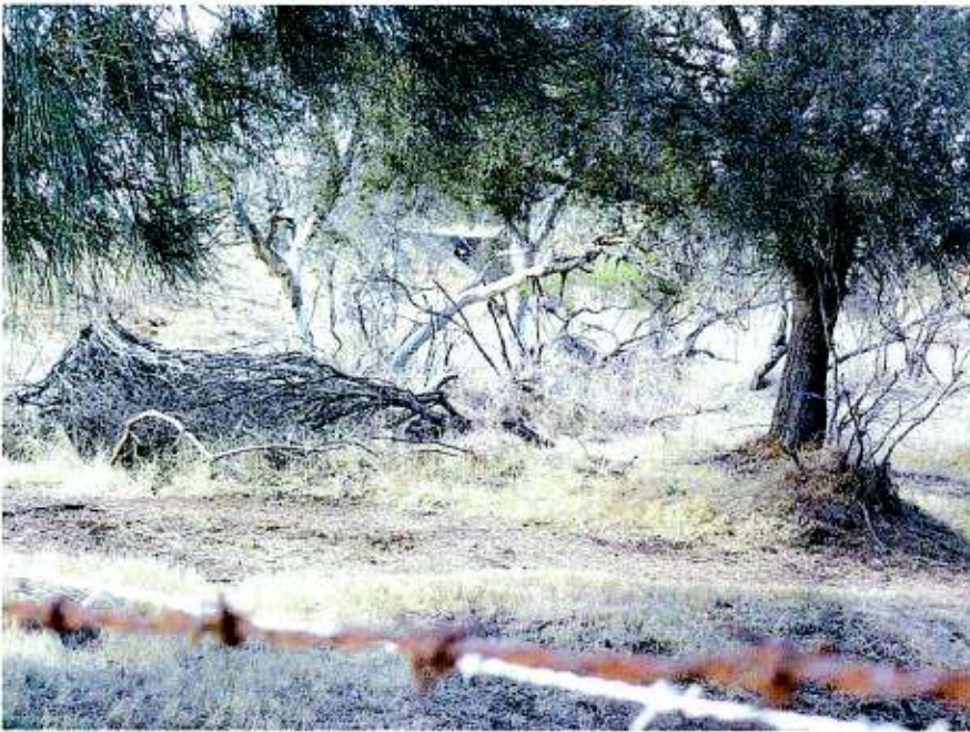
View looking southeast showing the culvert in the side of the alignment formation. April 2010.
