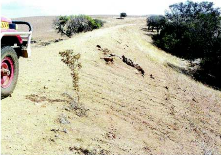
NORTH of the SUBJECT AREA. Approximately 1 kilometre north of the intersection of Olsen and Oakajee Roads showing the railway formation - culvert at base of tree on left- both sides. April 2010
